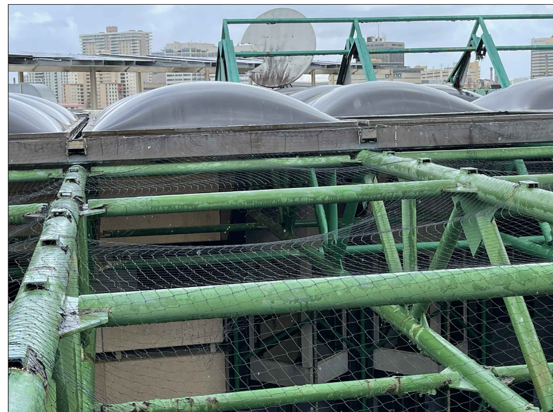
TYPICAL EXAMPLE OF FINDING ON TOP OF TRUSS.
