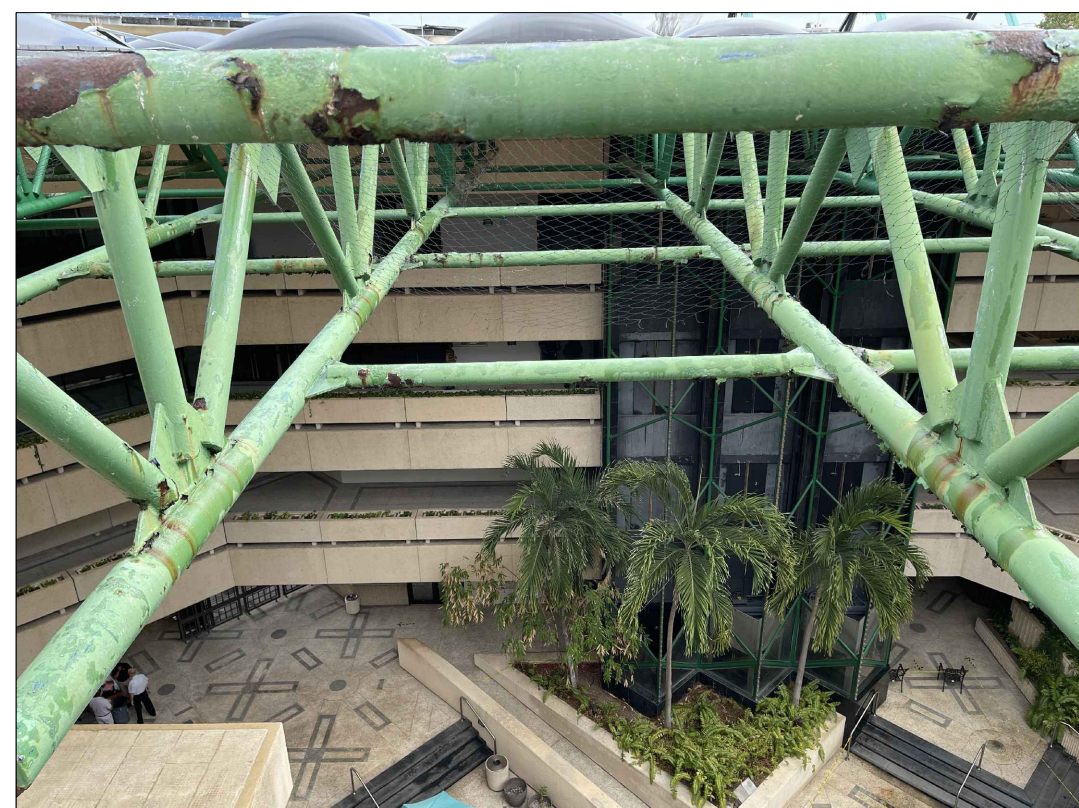
TYPICAL EXAMPLE OF FINDING ON BOTTOM OF TRUSS.
