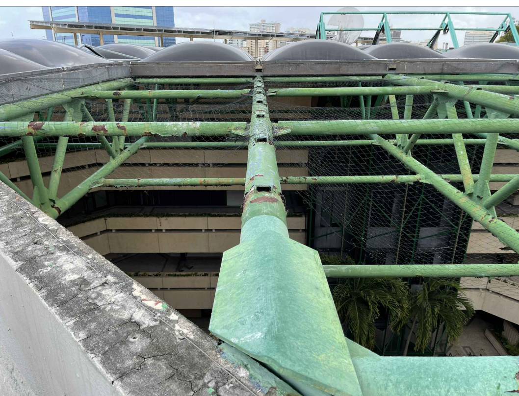
TYPICAL EXAMPLE OF FINDING ON TOP OF TRUSS.
