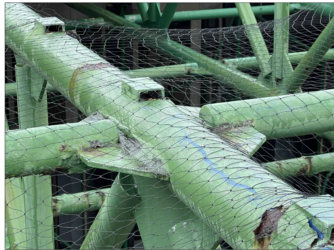
TYPICAL EXAMPLE OF FINDING ON TOP OF CONNECTION.
