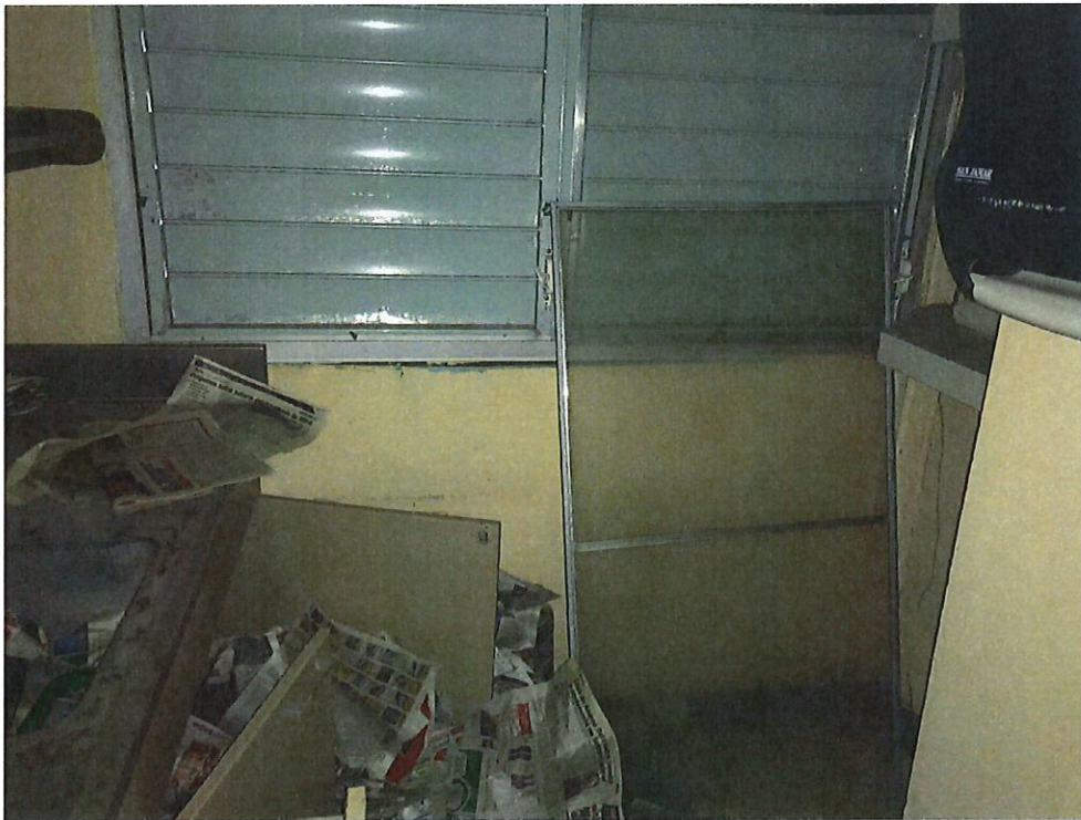
Photo Number 19 – Wall Interior "A" Clean Utility
