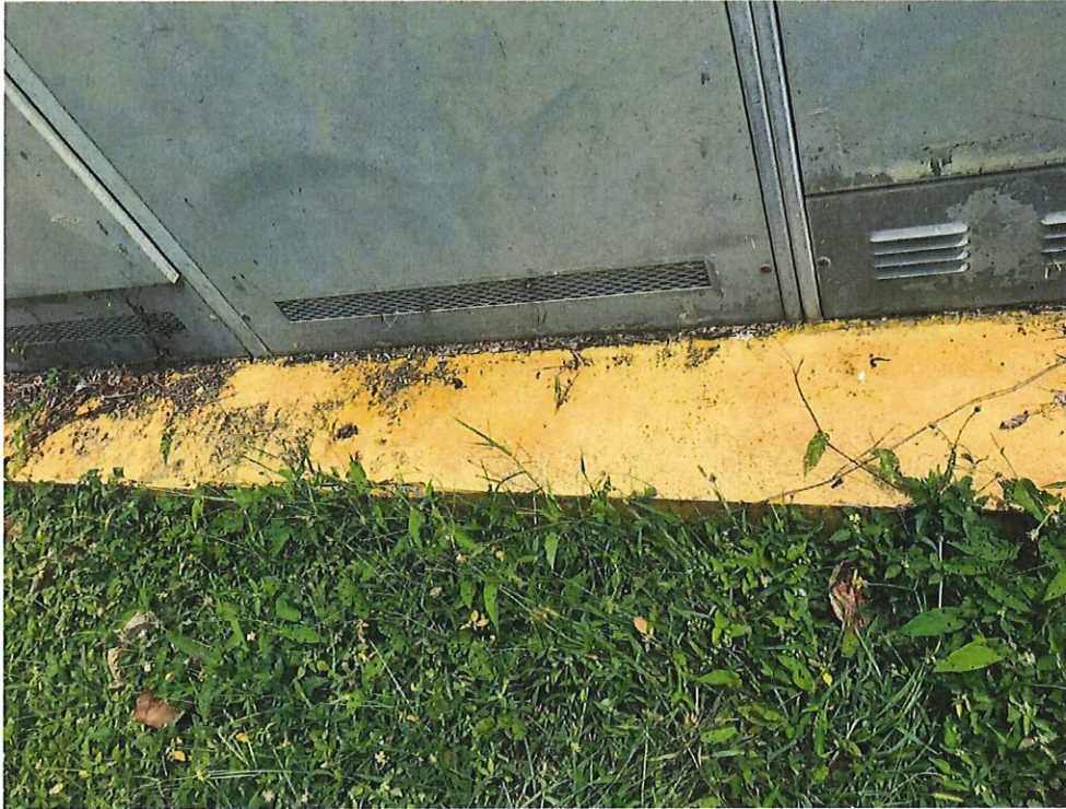
Photo Number 35 – Building Exterior Electric Transformer Slab
