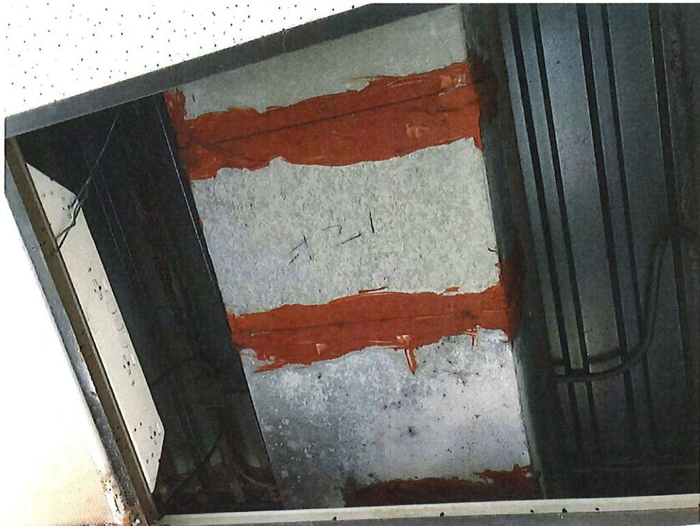
Photo Number 7 – Exam & Treatment Room Red Mastic Duct Air
