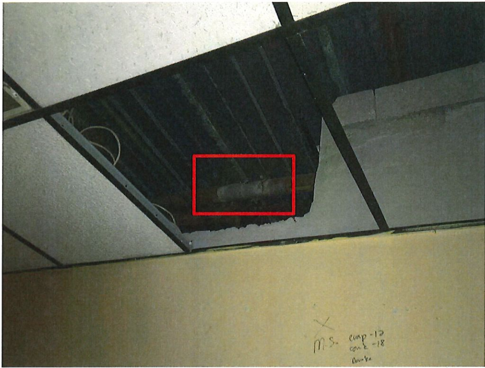
Photo Number 12- Hot Water Return Pipe Insulation
