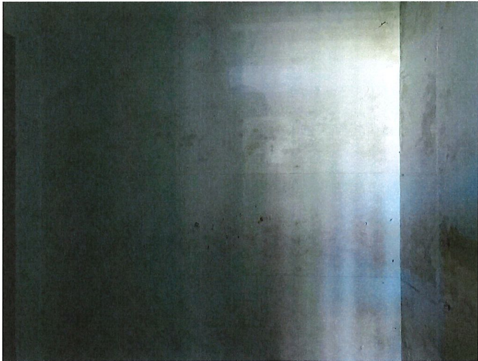
Photo Number 12 – Wall Interior “C” Dark Room at the X-Ray Room Area
