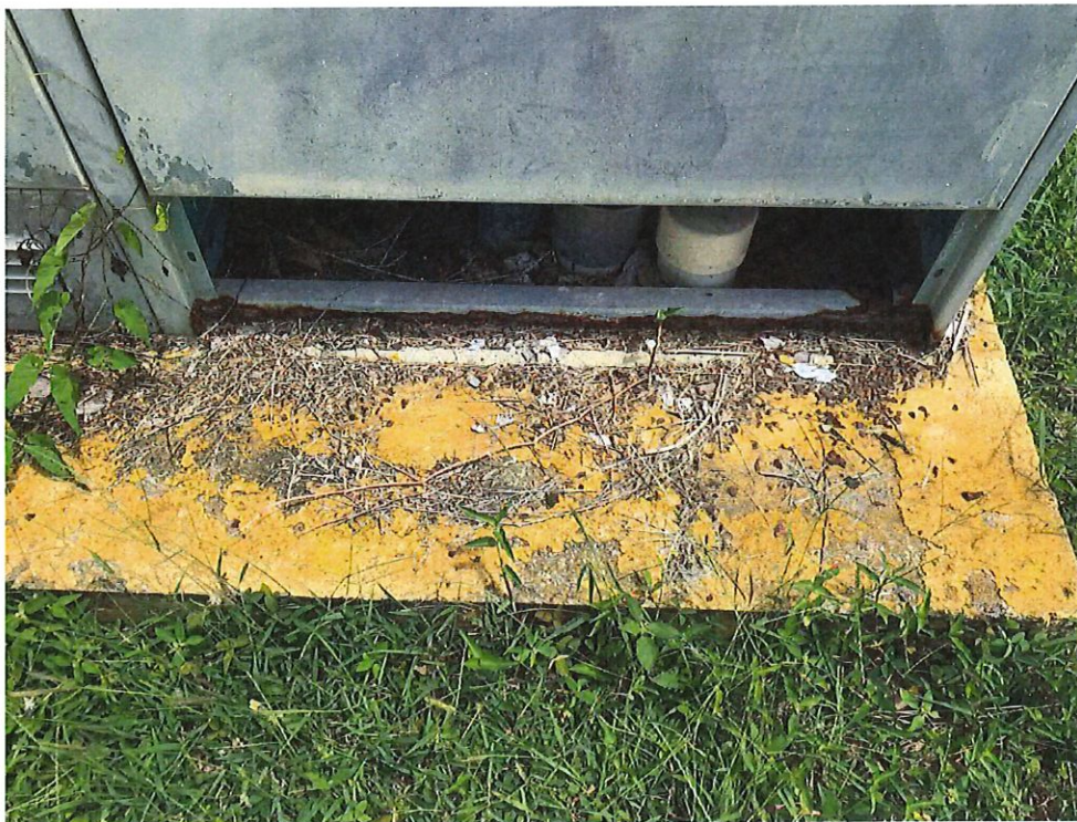
Photo Number 34 – Building Exterior Electric Transformer Slab
